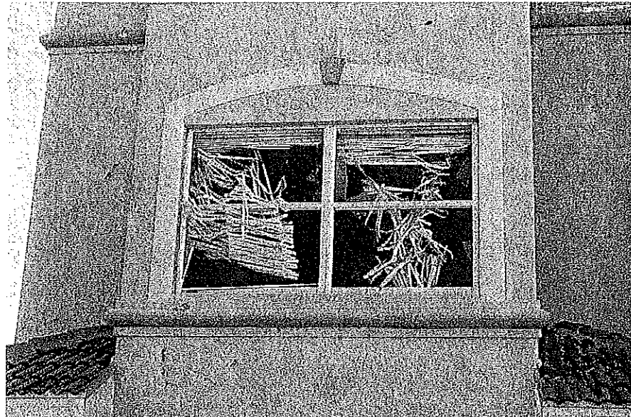
Window Glass Broken from Windborne Debris
