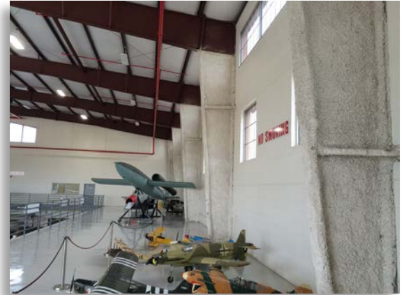
In some occupancies, spray-on fire-resistant material is not required for roof structural protection above 20 feet (6 meters). (Photo/Byron Blake)
