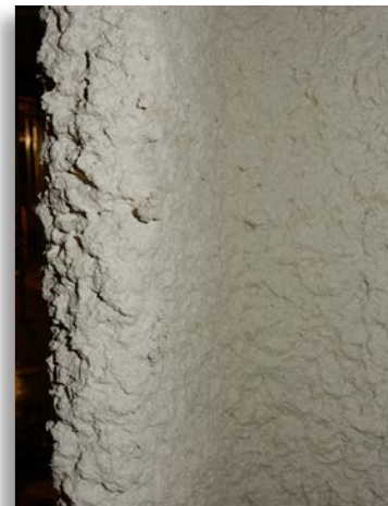
The thickness of spray-on fire-resistant materials must be inspected and documented to ensure that it meets hourly fire resistance rating requirements.
